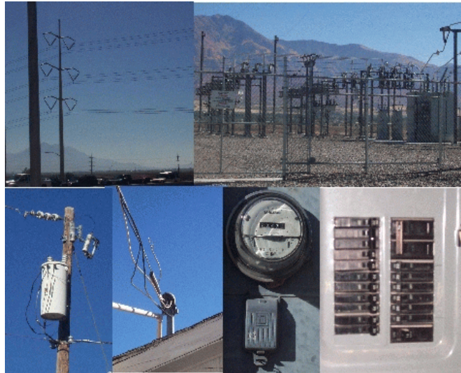
Figure 13.7. The route of electric power into a home: high voltage power lines, substation, transformer, service drop, electric meter, service panel (circuit breakers).
